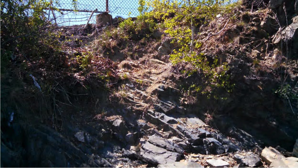
Photo 7 Proposed revetment 1 - ongoing erosion.
